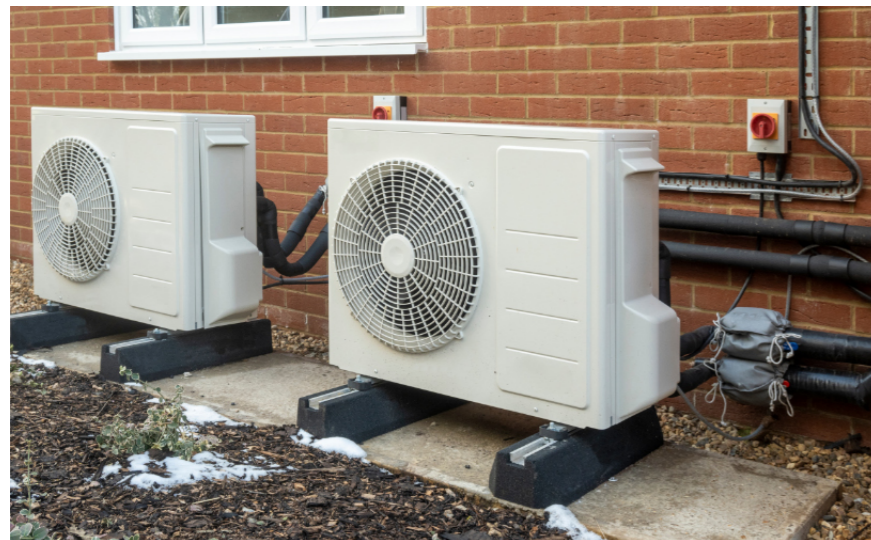
Figure 9: An Air Source heat Pump
