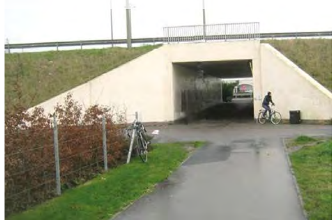
Figure 10.51 Underbridge near Cowley on Oxford Bypass with at-grade approach, wing walls and clear sightlines
