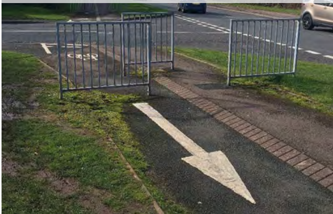
Figure 14.3: Poor quality provision for cycling in a housing development – no priority at side road, compounded by barriers
