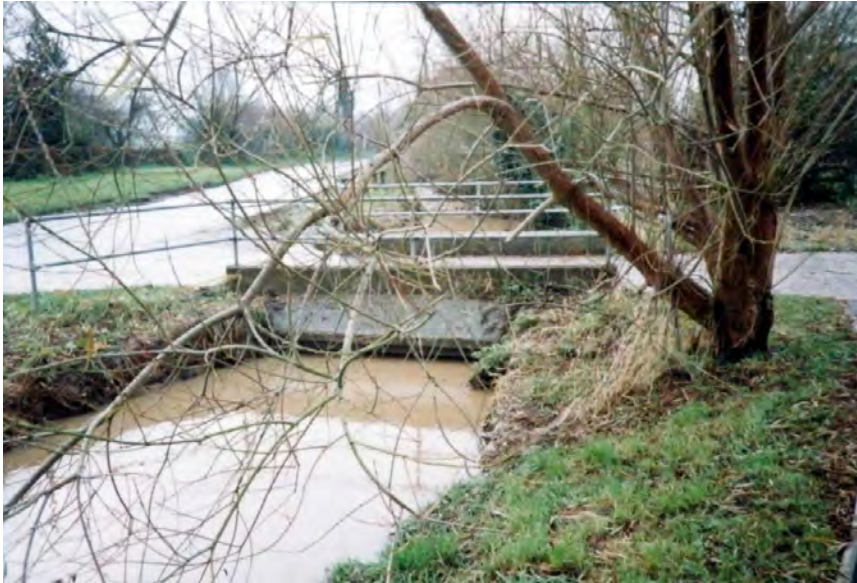
Photograph 2. Water level rising to parapet of occupation bridge on Moor Lane
