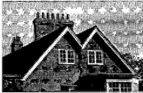
Figure 21 – Double pitched roof, large chimney stack and curving down pipe of Clifton Manor
