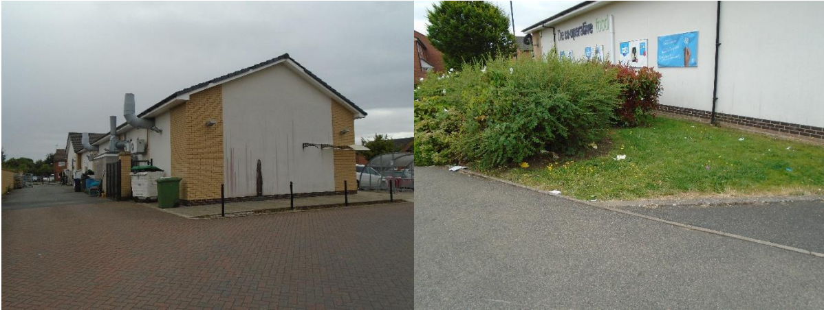
Left: Western elevation of the retail building with an unattractive view of the rear, stained render, and a damaged awning. Right: Shrubs on the east of the Co-op where noticeable amount of litter is collecting.
