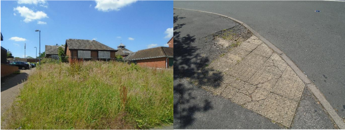
Left: The vacant building which formerly housed the doctor's surgery. Right: Example of paving in need of repair.
