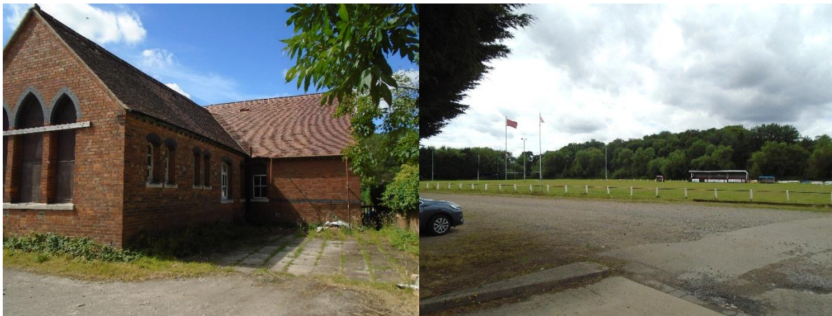
Left: View of the rear of Newbold Village Hall showing slipped roof tiles, faulty rainwater goods and boarded windows. Right: The extensive grounds of Newbold on Avon Rugby Football Club.
